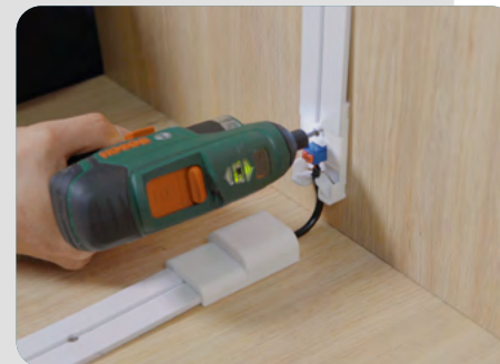
INSTALL A BYPASS
